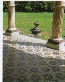
For the floor of the veranda, tiles with a design motif reminiscent of traditional Islamic designs were used.
